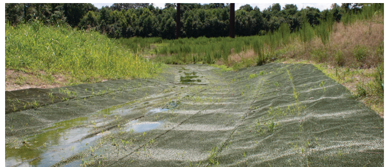
After hurricane—outfall channel.
