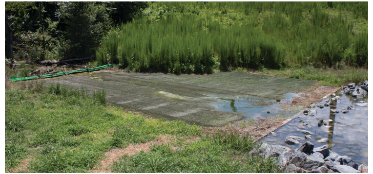
After hurricane—emergency spillway.
